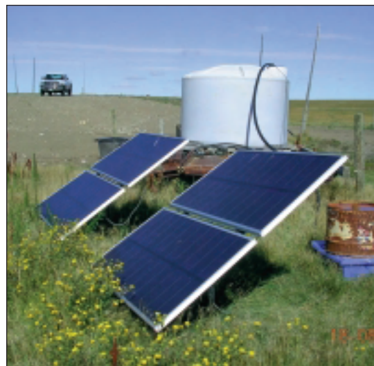
Solar panels and holding tank
