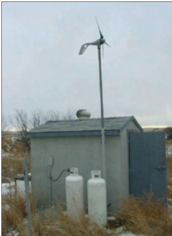
Propane tanks and windmill system.
