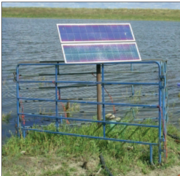
Panels and pump, situated at edge of marsh
