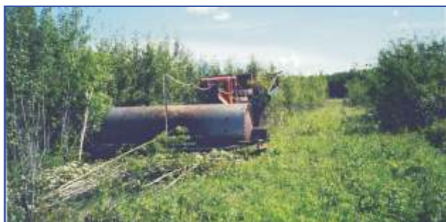
Smooth drum on a demonstration project at Ashville, Manitoba, 2002. Photo: Bill Gardiner
