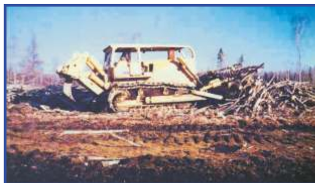
A bulldozer “walks down” the trees and pushes them into piles. Photo: Bill Gardiner
